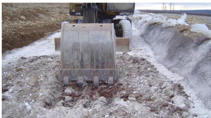
Fig. 1. The work on strengthening the soils on karst land of the railways in Yakutia.
