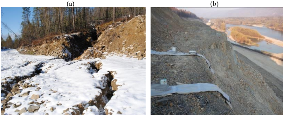
Fig.1. The top of the slope and the longitudinal cracks (a); GPR acquisitions on the steep slope (b).
