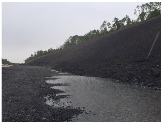
Fig. 1. Watered area at the cut slope bottom.
