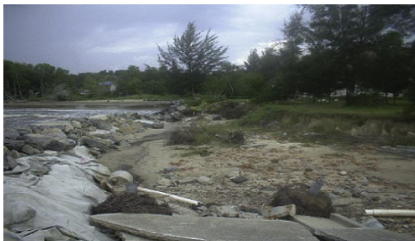
Fig. 8. Failure of protection measure protection.
