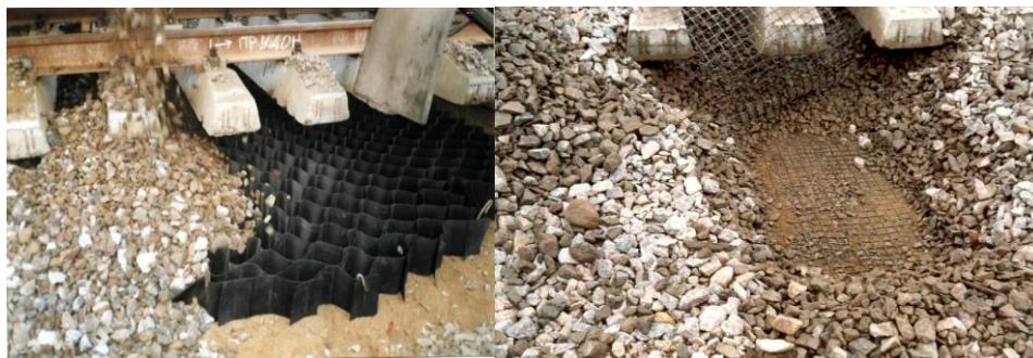
Fig. 3. Laying of geocells and two geogrid layers on the top of subgrade.
