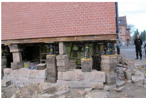
Fig. 1. Example of wooden supports installed in the wall of the straightened building
