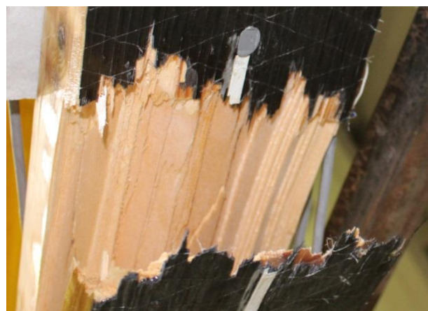
Fig. 12. Rupture of carbon fibres of BCLT50 beam.
