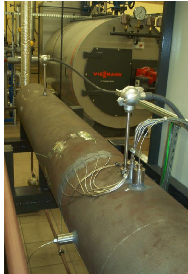
Fig. 4. View of the instrumented steam header before the foundation of the thermal insulation
