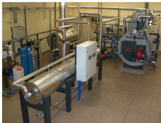
Fig. 1. View of the experimental installation for testing the computer system for on-line monitoring thick-wall pressure components
