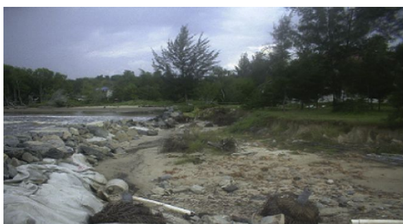
Fig.14 Failure of protection measure protection
