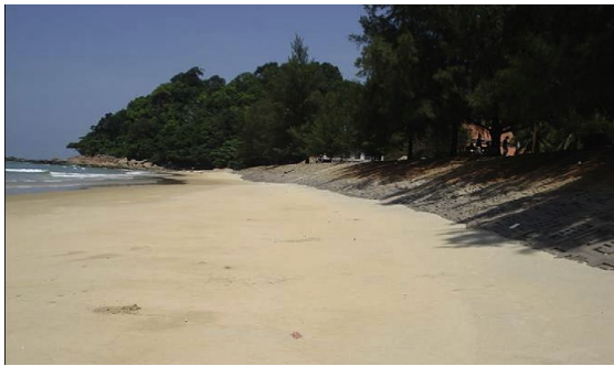
Fig. 18 The condition of shoreline and beach in December 2009 after completion of submerged geodykes installation
