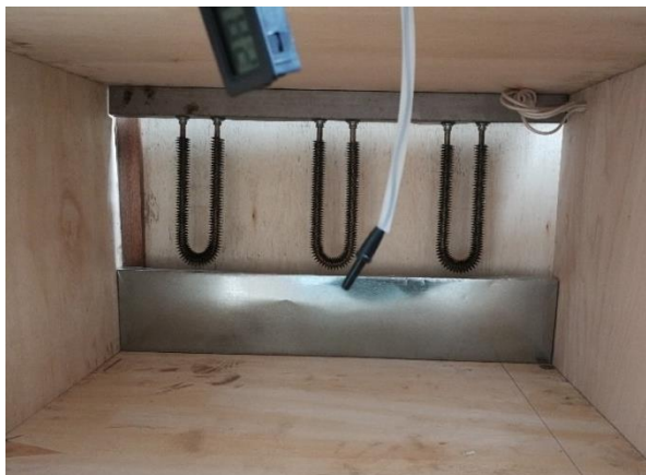
Fig. 4. Three stages of coil heater installed in the outdoor unit's ductwork.
