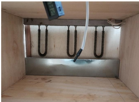
Fig. 2. Three stages of coil heater installed in the outdoor unit's ductwork.
