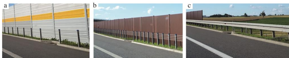
Fig. 1. An example of a) the local change in post spacing, b) the missing post in cable barrier c) the missing post in steel barrier.
