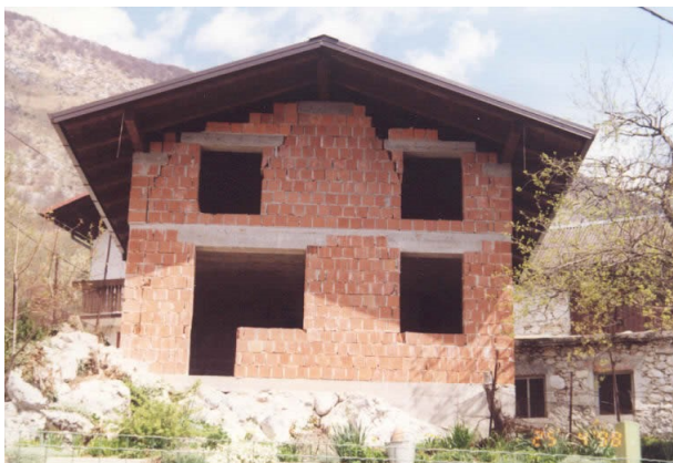
Figure 6 Typical earthquake damage: a house without vertical tie-columns and without top bond-beams in Attics (1988 Bovec earthquake) [31]
