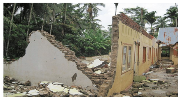
Figure 4 Buildings in Padang, Indonesia after earthquake September 30, 2009 (7.6 on Richter scale). Damages to an unconfined single story school building [29]
