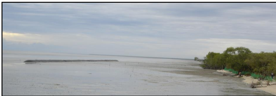
Fig. 1b. The sand-filled, wave breaker (geotubes), constructed at the beach of D’ Muara Marine Park Resort, Sungai Hj Dorani, Selangor (before planting) in July 2007
