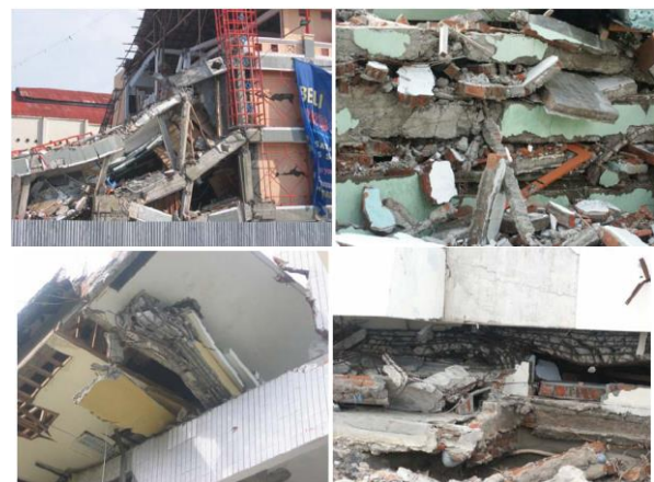
Fig. 1. 2004 mega earthquake damages at Banda Aceh [2].
