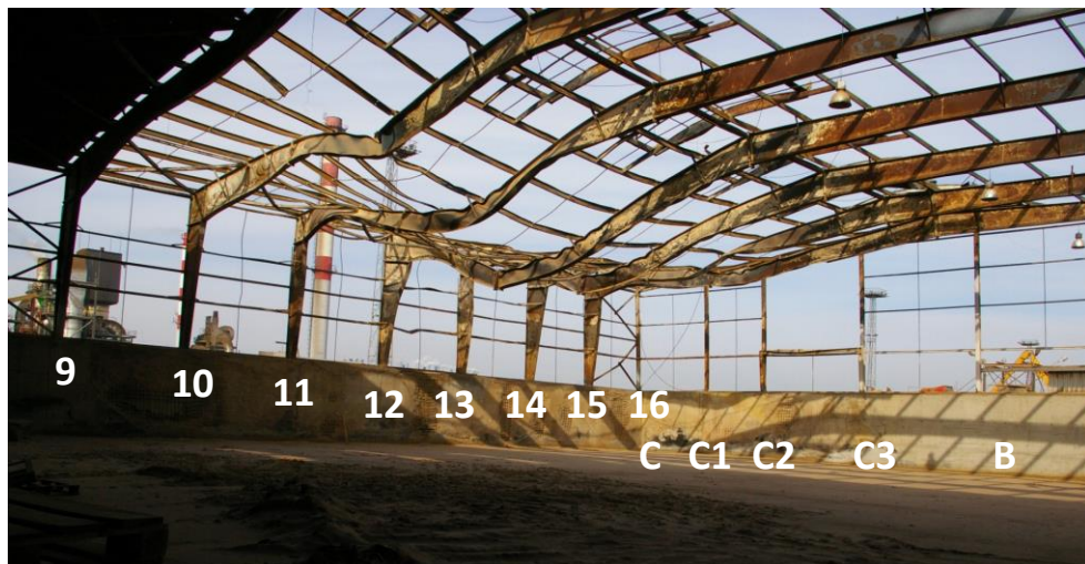
Fig. 4. Deformation of the steel structure between axis B - C and 9 – 16.
