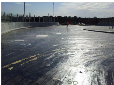
Fig. 2. Membrane failure in a deck area with the signs of bubbling.
