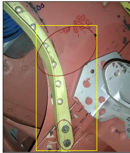
Fig. 10 Crack near the reinforcement plates
