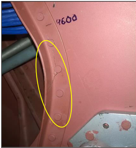
Fig. 9 Cracks near the stiffener to replace
