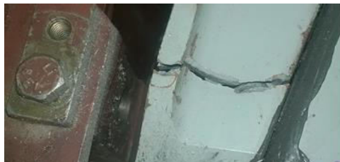
Fig. 11 Failure of hinge console
