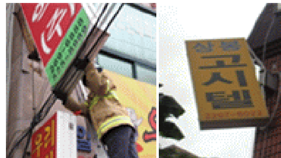
Fig. 1. Failure of sign structure.
