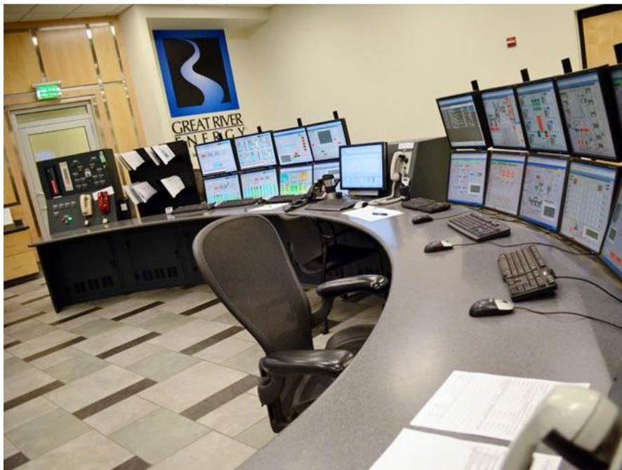
Fig. 1. Power Plant Control Room view.
