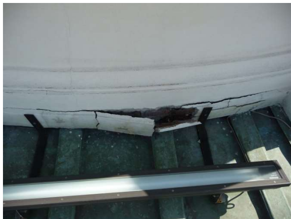
Fig. 4. Cracks of cornices and cracks on the facade of the dome of the church of St. Anne in Wilanów.
