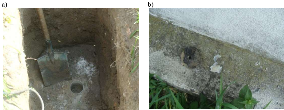
Fig. 4. A vault over the damp rooms of the building No. 36; a) the visible the test bore-hole of the wall after drilling b) insulation layers discovered (tar paper and zinc sheet).
