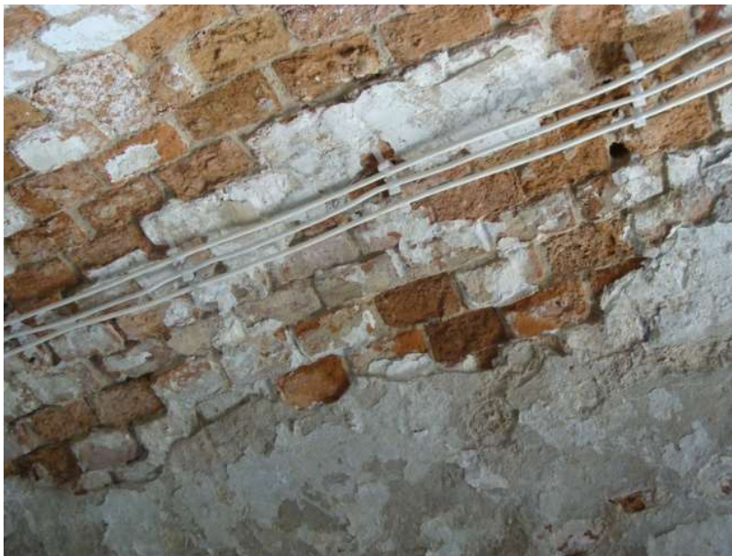
Fig. 5. Blistering of wall covering and spalling of masonry construction in rooms of facility No. 60.
