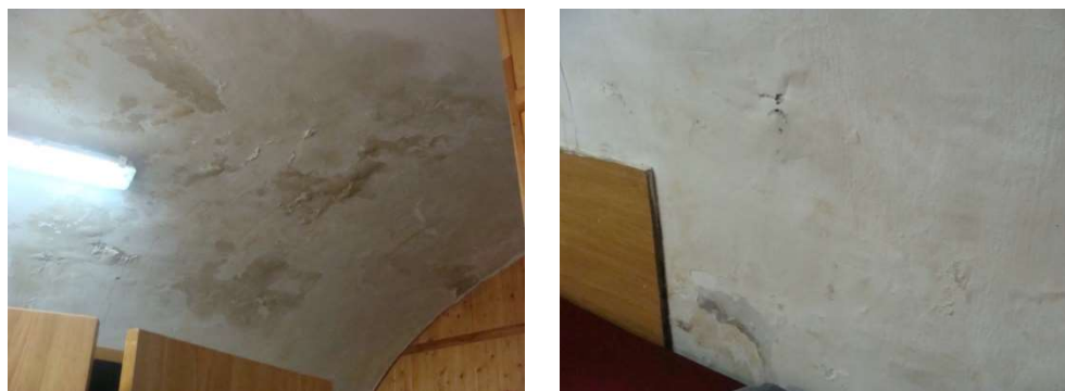
Fig. 3. Moisture accumulated on the ceiling vault in the building No. 36.
