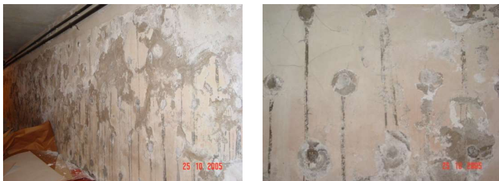
Fig. 1. “Salt damp” damage observed (fretting mortar, bubbling paint and plaster, as well as serious decomposition of the wall materials) on the rear wall of the eastern outbuilding in the basement. Visible places of holes in the wall made during the drying works using the crystalline injection method.
