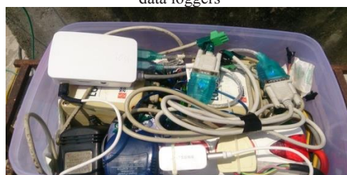
Figure 5. Connections inside the box
