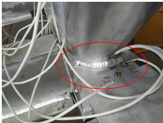
Photo 2. Node with a propagated fatigue crack
