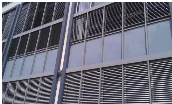
Fig. 2. An example of a simple sun shield on the outer surface of the wall in a temperate climate (Berlin, Germany. Photography from a personal archive of authors).
