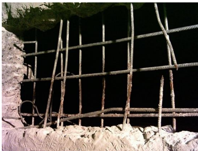
Fig. 2. Corrosion damage to reinforcement with a loss of rebar cross-section up to 80%.
