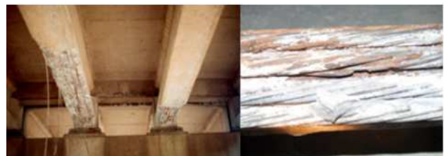
Fig. 1. Corrosion of the prestressing steel [2]
