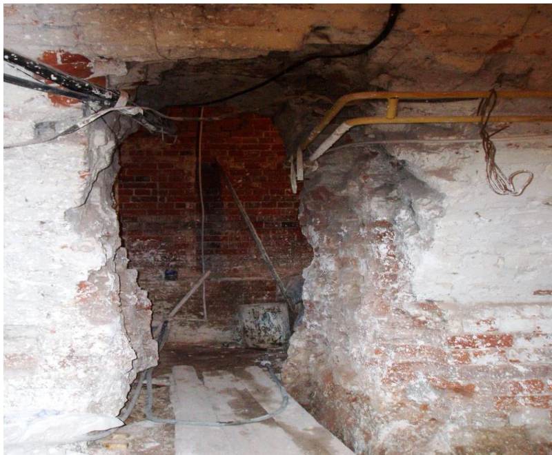
Fig. 1. Type of load-bearing structures of the Cathedral of St. Alexander Nevsky, exposed to moisture, before reconstruction.
