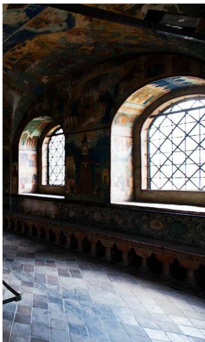
Fig. 2. The walls in the ancient unique buildings have a thickness of more than 1 m.
