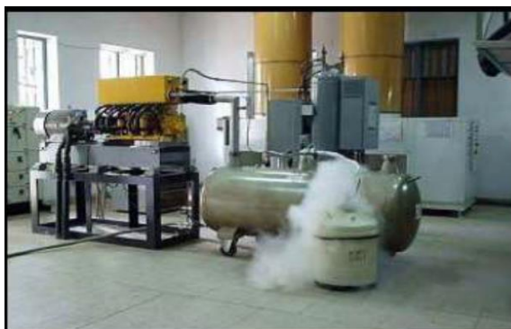
Fig. 1. Cryogenic Treatment Equipment
