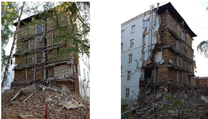
Fig. 4. The real collapse of the northern block of the building.
