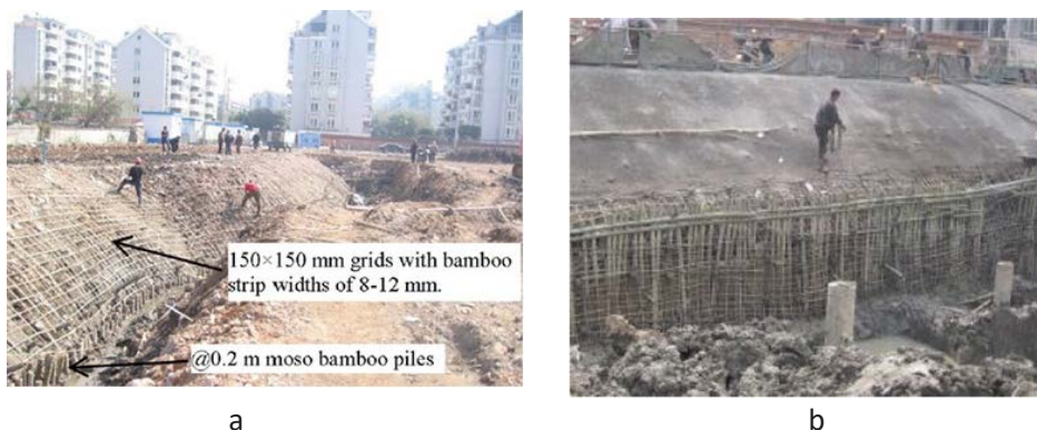
Fig. 5. Combination of bamboo soil nails, bamboo sheet piles, and bamboo reinforced shotcrete for slope stabilization (adapted from [16, 17]).
