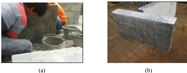
Fig. 4. Process of making specimens of hollow core concrete brick wall: (a) organizing the hollow concrete bricks, (b) hollow core concrete brick walls
