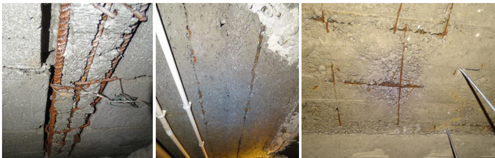
Fig. 3. Reinforcement not protected since construction moment (photos by Piotr Knyziak, 2016)
