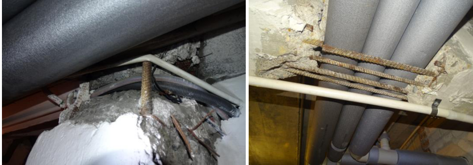
Fig. 4. Reinforcement exposed during installation work and not secured (Piotr Knyziak, 2016)
