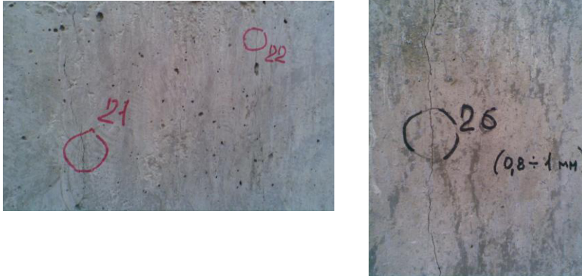
Fig.4. Cracks on the outer surface of PC.
