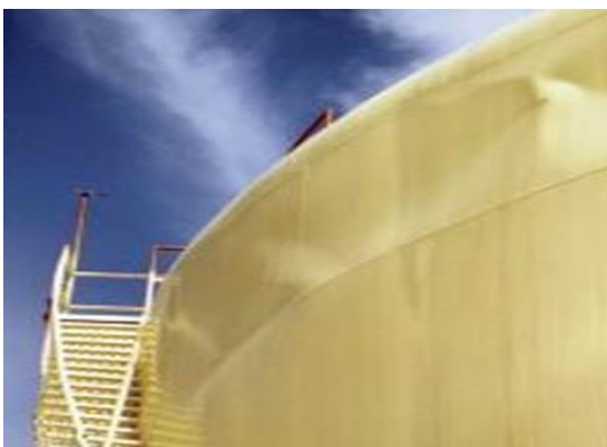
Figure 1. Damage on the roof of a tank after excessive sloshing liquid content.
