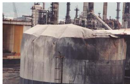
Figure 2. Activation of a fire in a tank in Turpas raffinery after Koaceli's Earthquake 1999 (Turkey).
