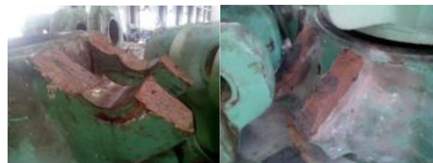
(a) Fractures of Lug Holes (b) Fractures of Lug Roots Figure 1. The Fractures of the Hinge Beam
