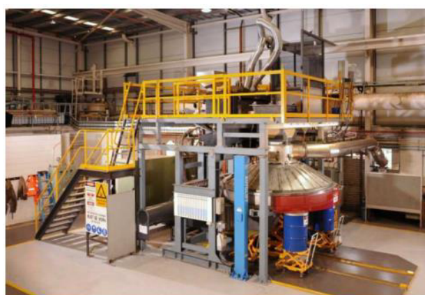
Figure 7. The semi-industrial scale (3 m in diameter) integrated heat recovery and dry granulation pilot plant at CSIRO with design throughput of 6 tonnes/hour of slag [8].
