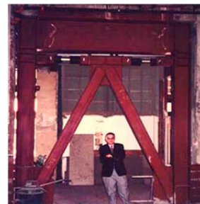
Damper installation in chevron bracing
