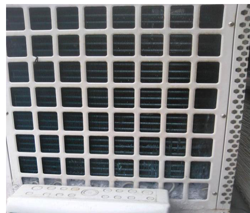
Figure 2. Evaporator After Defrostation
