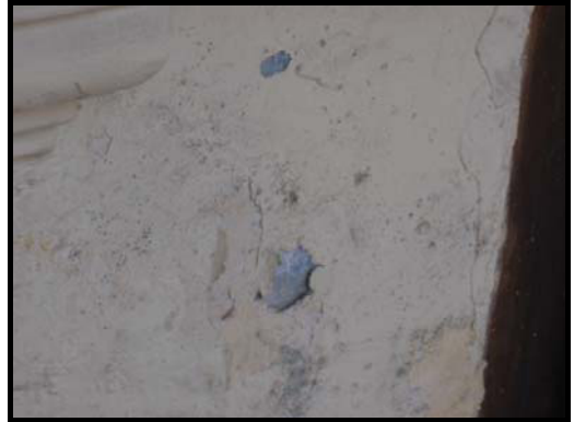
Fig 7: Peeling paint on exterior wall
