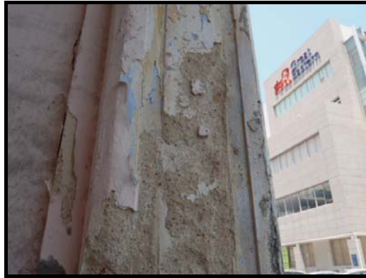
Fig 4: Wall deterioration due to the use of incompatible materials.
