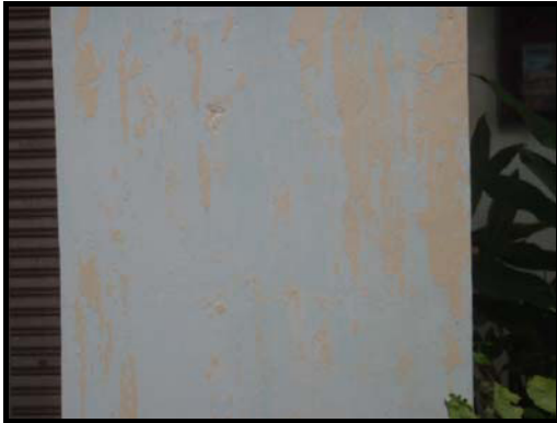
Fig 6: Discolouration on a wall
