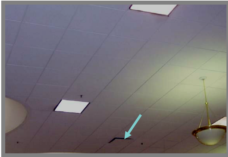
Figure 1. Ceiling in Baling Bayu Engineering shows the loose sheet of ceiling
