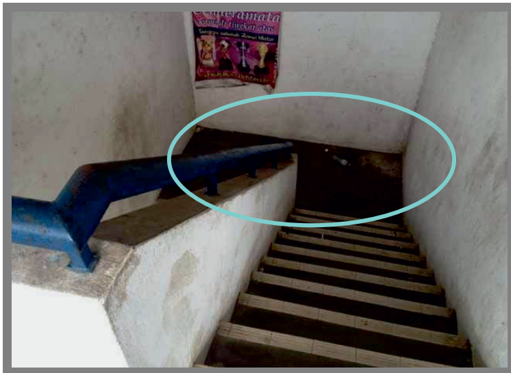
Figure 2. External cleanliness at one of the offices – animal faeces on the floor
