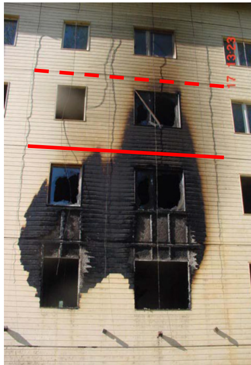
Figure 2. Damages of the wooden façade after the natural fire tests in Merkers [4] and difference of safety goals between Austria and Germany (dashed line).
