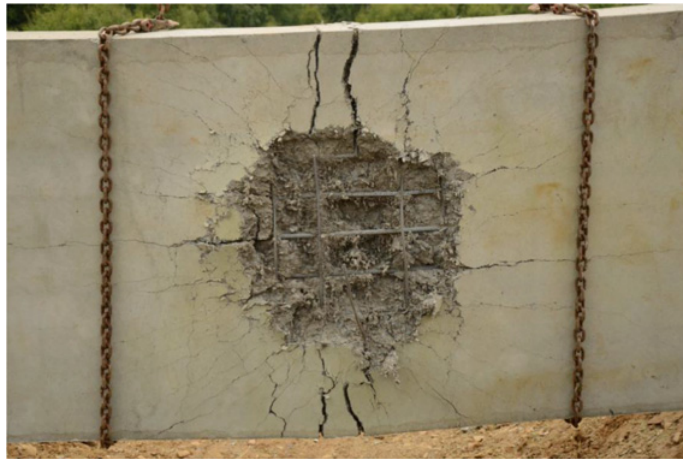
Figure 3. Damaged specimen No. 5 (FRC) after blast – bottom view.
