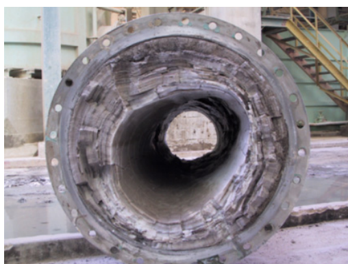
Figure 1. Precipitation of compounds containing salts of Hexafluorosilicate on the pipes during the production of phosphoric acid.
