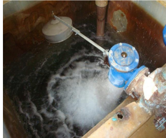
Photo 2. Photo of potable water tank and water charge breeze before intervention.
