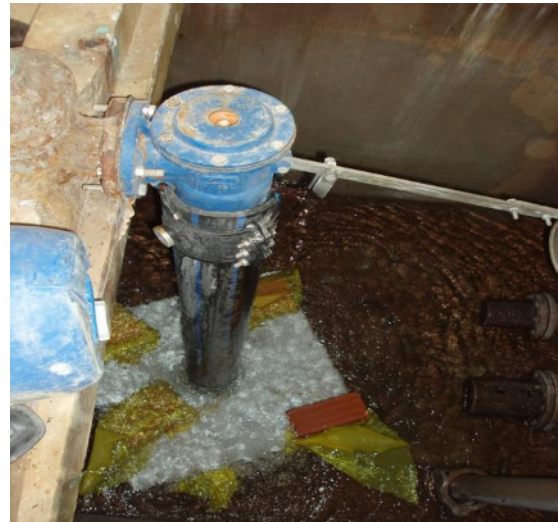
Photo 3. Photo of potable water tank and water glances of venting after intervention.
