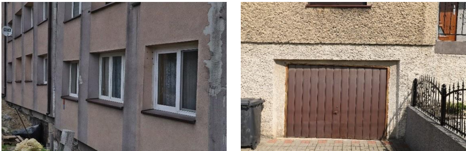
Fig. 4. An example of windows and doors in deflected buildings.
