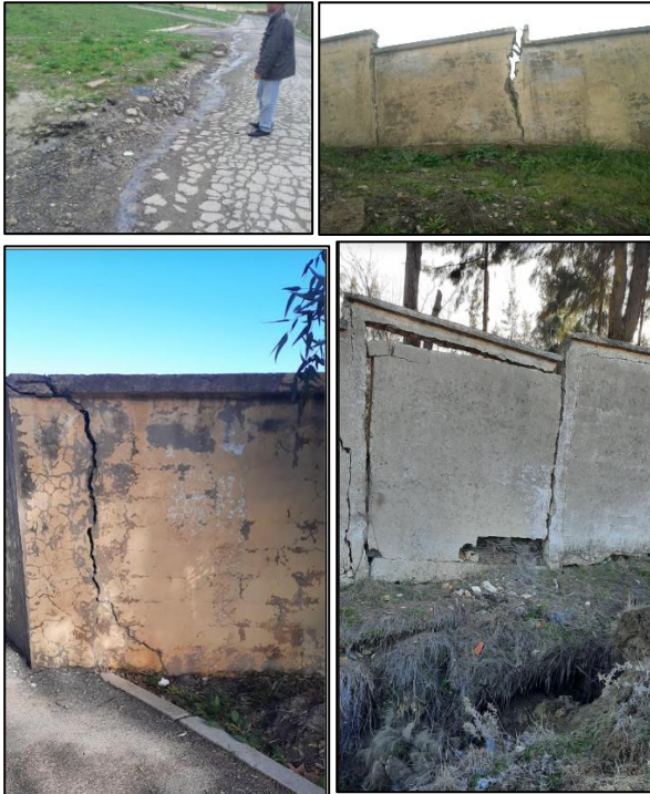
Fig. 1. Damage to boundary walls, footpaths, pavements, and hydraulic installations as a result of the shrink-swell cycle in the Medea region.
